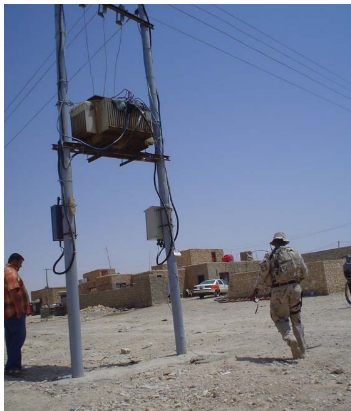
A local contractor and an engineer with a Civil Affairs team from the 96th Civil Affairs Battalion (Airborne), Fort Bragg, N.C. inspect the recently installed transformer and power lines in the village of Al Ashoudalaa, Iraq. This rural project brought electricity for the first time ever to more than 500 families in a remote village in Al Anbar Province, Iraq. U.S. Army photo.
