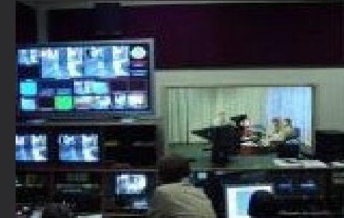
MPC-H Control Room
